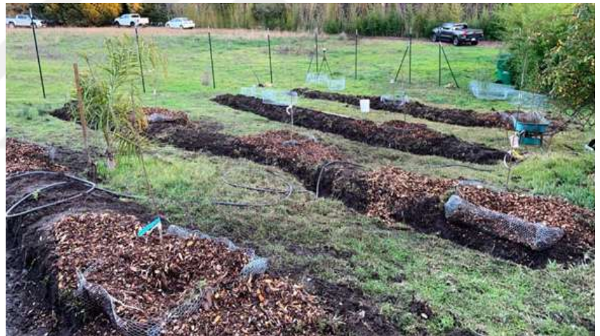
Figure 97. (Top) A sketch for building a rain swale. (Bottom) An example of field implementation of the rain swale. (Santa Cruz Permaculture Community)
