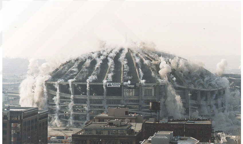
Figure 53: Implosion of the Kingdome, (Source: Sarah Anne Lloyd, 'The Kingdome imploded 18 years ago today', Curbed Seattle , 26 March 2018,)
