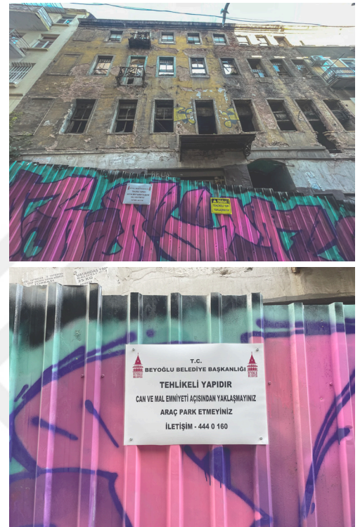
Figure 38: Enclosed Building, “Dangerous Structure” Warning
