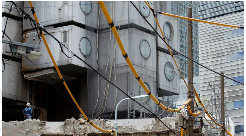
Figure 10: Demolition of Nakagin Capsule Tower (Source: James Parkes, "Footage reveals dismantling of Nakagin Capsule Tower in Tokyo", Dezeen, 29 April 2022, https://www.dezeen.com/2022/04/29/nakagin-capsule-tower-demolition-video-tokyo-japan/ ).
