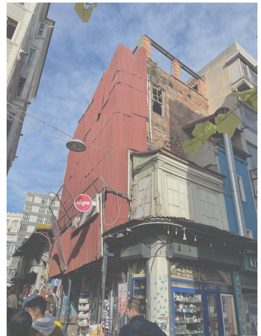
Figure 31: Building enclosed with aluminum which are rusted over time, Kardeşim St., No: 5A
