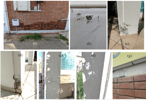
Figure 22: Building Pathology Study: (a) rising damp and salt crystallization damage to the fired red clay solid brick facade, (b) plaster detachment on painted infill walls, (c and d) plaster detachment on columns, (e and f) longitudinal cracks due to corrosion of the reinforcement, (g) vertical crack at the center of the entrance beam. (Source: Seismic assessment of historic concrete structures: The case of Pedieos Post Office in Nicosia, Cyprus)
