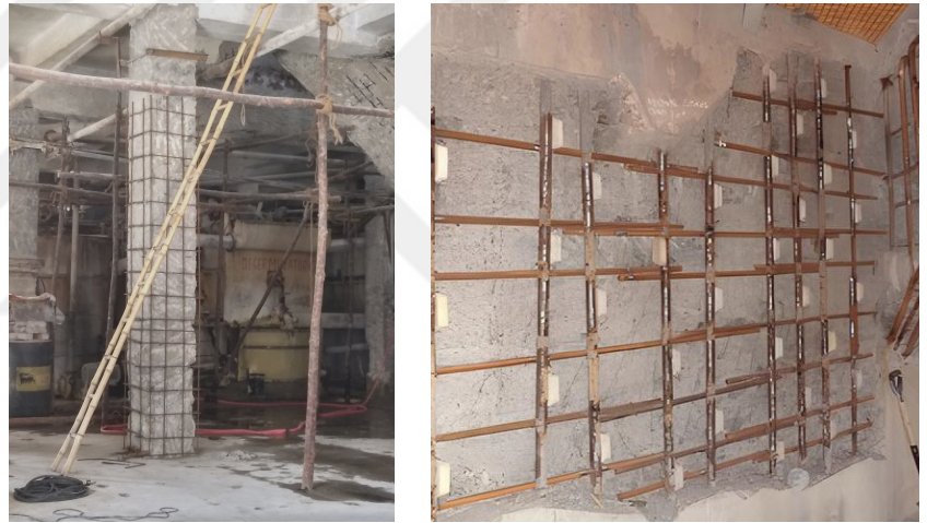
Figure 39: Deep repairs for corroded reinforcements in the existing structure. (Left: IndiaMart, "Building Rehabilitation Repair Work, In Industrial", Right: Csc Services, "Concrete Repairs Cathodic Protection".)
