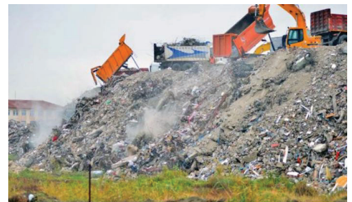
Figure 1: Demolition debris, Mileyha Wetland, Hatay, Türkiye 2023 Source: Haber Global
