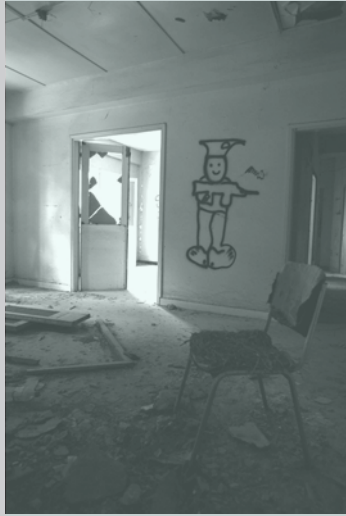
Figure 7: A view from one of the residential units on the upper floor, showing the interior condition.
